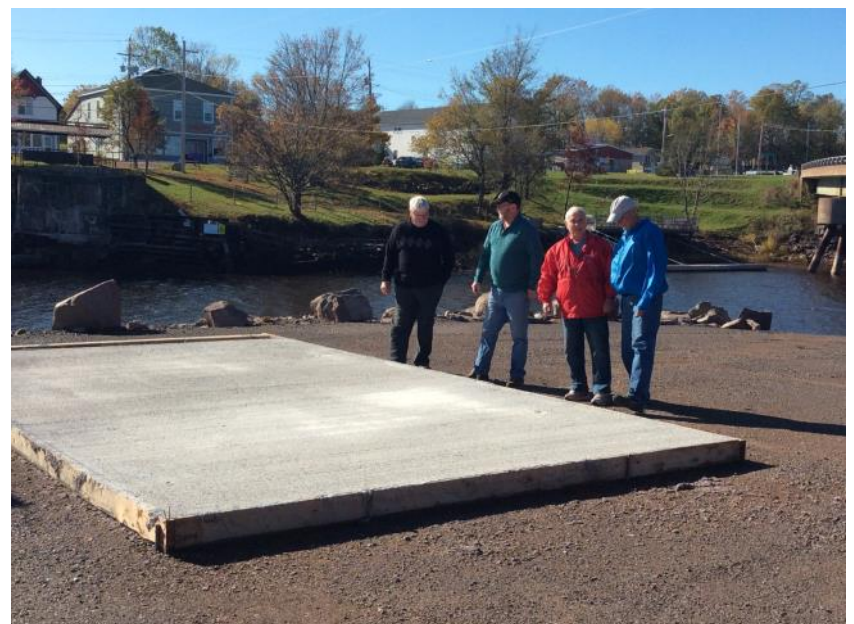
This concrete slab will be moved to form the slipway into the water.
